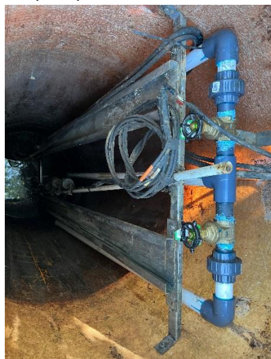
New pump shutoff valves
