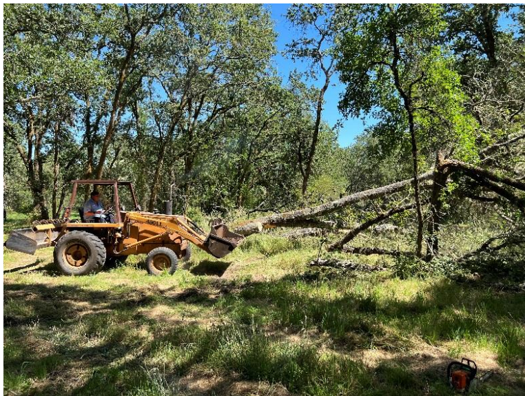
Operators pulling away the fallen tree from a broken riser
